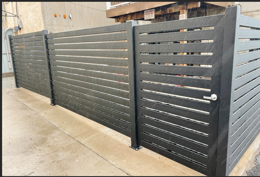
CUSTOM MADE PRIVACY WALL WITH DOOR FOR DOWNTOWN CASTLE ROCK
